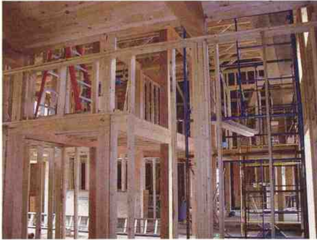
In early March, the new interior only hinted at the shape of offices to come.
