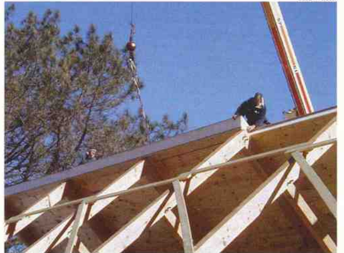
The VTFC crew was halfway through laying down the new roof by President's Day.
