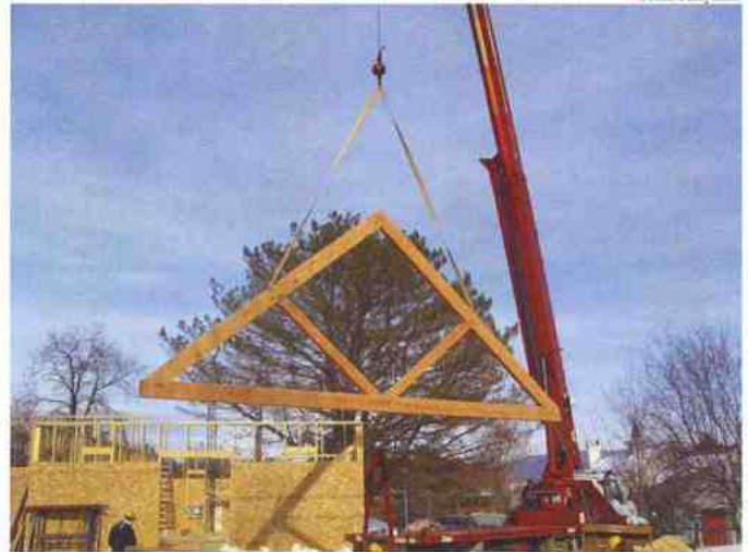
In early February, the Vermont Timber Frame Company began work on the gallery roof, using a massive crane to lift pieces of the framework into position.
