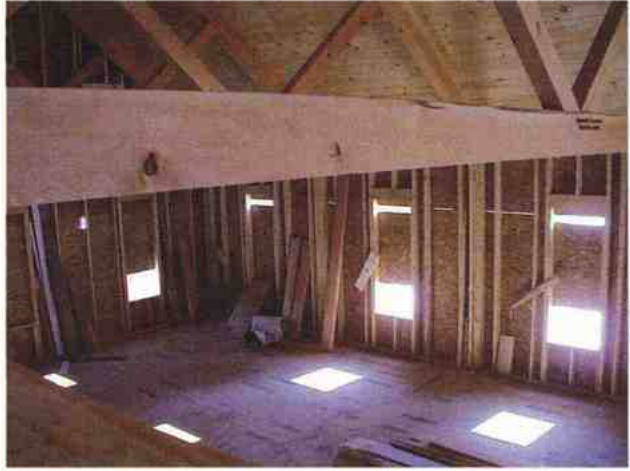
A look at the future gallery as seen from the second floor.
