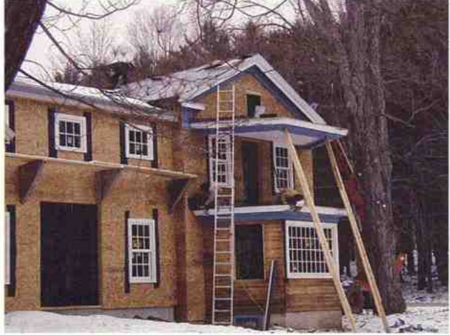
By late March, the construction crew installed windows and began work on both the new and historic portions of the roof.
